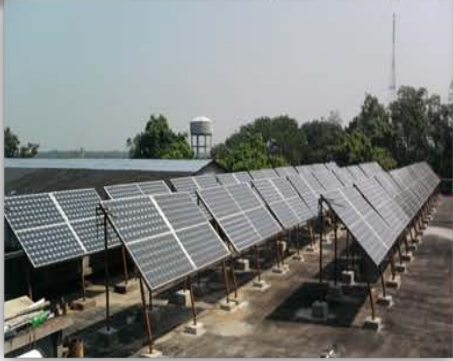
SOLAR PV ARRAY (Primary Source)
