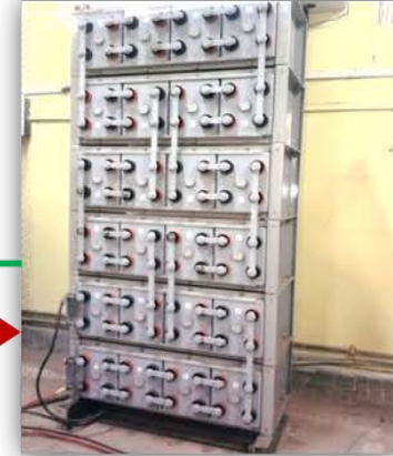
BATTERY BANK (Back Up Source)
