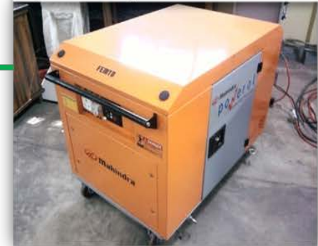
DIESEL GENERATOR (Back Up Source)
